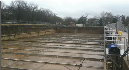
Dalecarlia WTP/Sludge Collectors – Washington, DC
