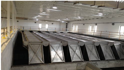
Utah Valley WTP/Plate Settlers – Orem, UT
