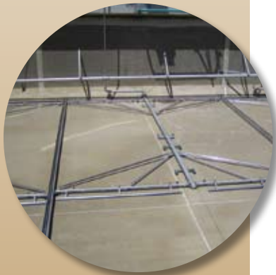
THE EL SOBRANTE WATER TREATMENT PLANT IN OAKLAND, CA INSTALLED 22 MRI HOSELESS CABLE-VAC SYSTEMS.
