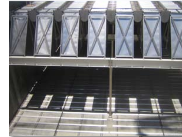
AT THE FACILITY IN BRISBANE, AUSTRALIA, MRI U/S ULTRA-SCRAPERS AND PLATE SETTLERS OPTIMIZE TERTIARY WASTEWATER TREATMENT.
