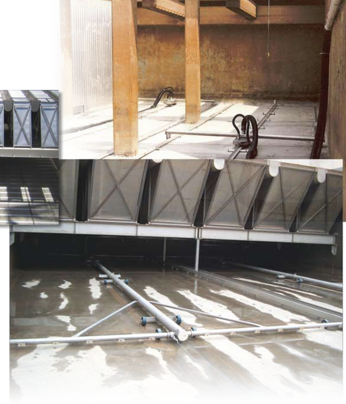
THE WATER TREATMENT PLANT IN PIEDMONT, AL WAS COMPLETELY REFURBISHED WITH THE MRI RETRO CABLE-VAC. (TOP) THE TOBACCO ROAD WATER TREATMENT PLANT IN AUGUSTA, GA UTILIZES THE MRI HOSELESS CABLE-VAC UNDER MRI STAINLESS STEEL PLATE SETTLERS. (BOTTOM)
