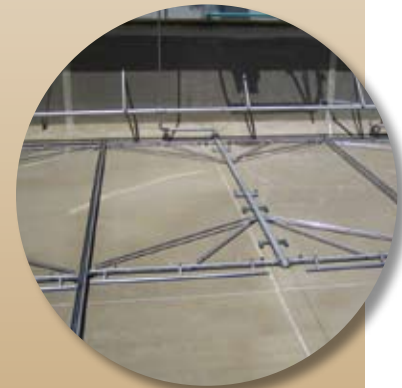
THE EL SOBRANTE WATER TREATMENT PLANT IN OAKLAND, CA INSTALLED 22 MRI HOSELESS CABLE-VAC SYSTEMS.
