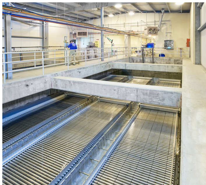
Red Mountain WTP featuring MRI Inclined Plate Settlers with "break-down style" cartridges and MRI Hoseless Cable-Vac Sludge Collectors.
