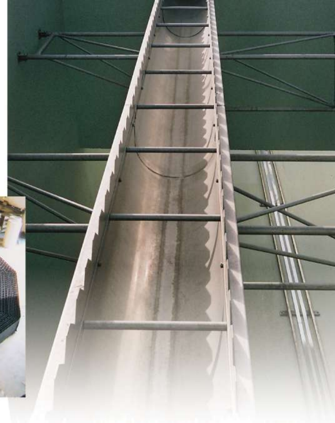
Pictured above: ARAMCO Water Treatment Facility, Saudi Arabia—Includes MRI round bottom stainless steel collection troughs and stainless steel supports.
